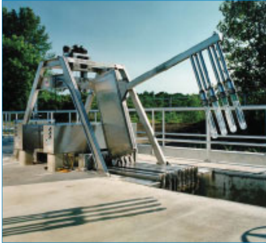
■ Fig 24. Waste water system.
